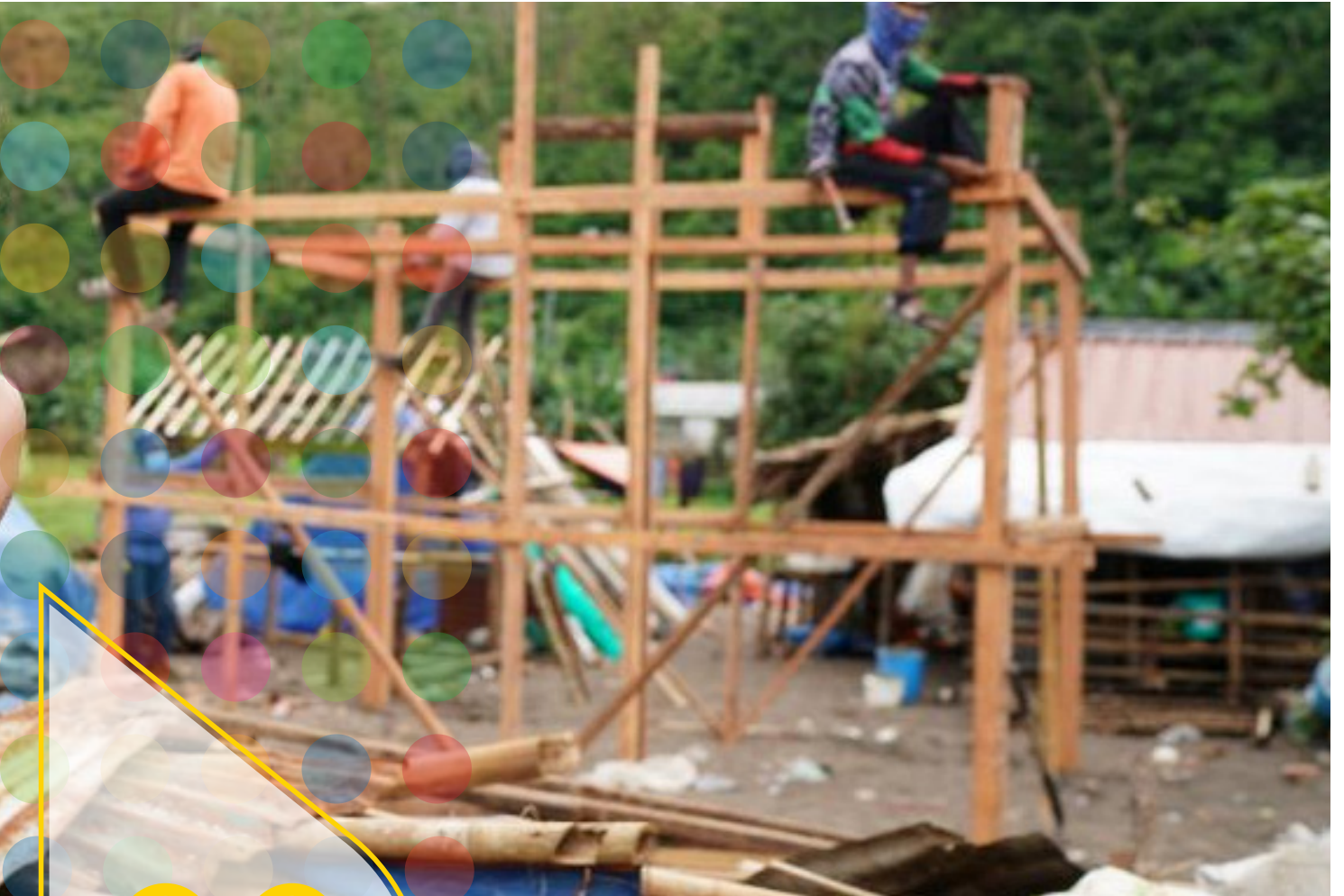
A family in Tiwi, Albay Province, rebuilds their home following the impact of Typhoon Goni through shelter repair assistance provided through Central Emergency Response Fund projects implemented by the UN Philippines. ©OCHA/ Martin San Diego
