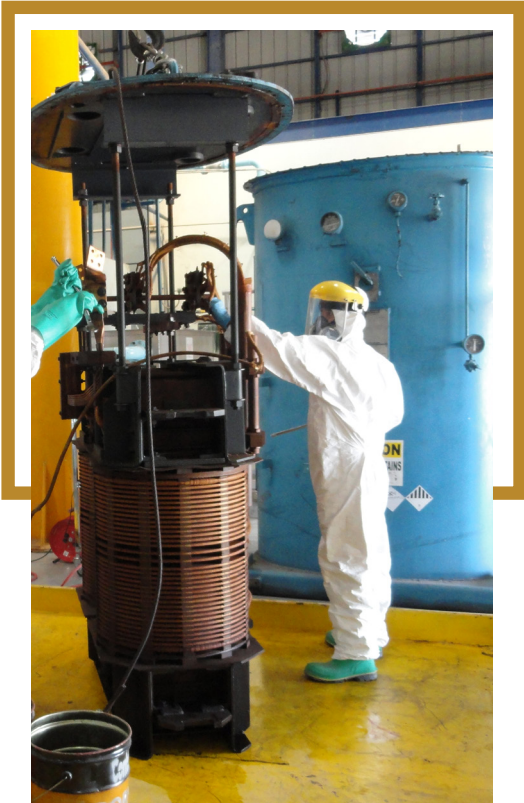
Decontamination of a power transformer at the Non Combustion Facility in Mariveles, Bataan. The plant was built to demonstrate the viability of available non-combustion technologies for the destruction of unintentionally released Persistent Organic Pollutants (uPOPs). © UNIDO/Edwin Punongbayan
